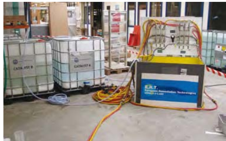
Fenton's pilot injection equipment
